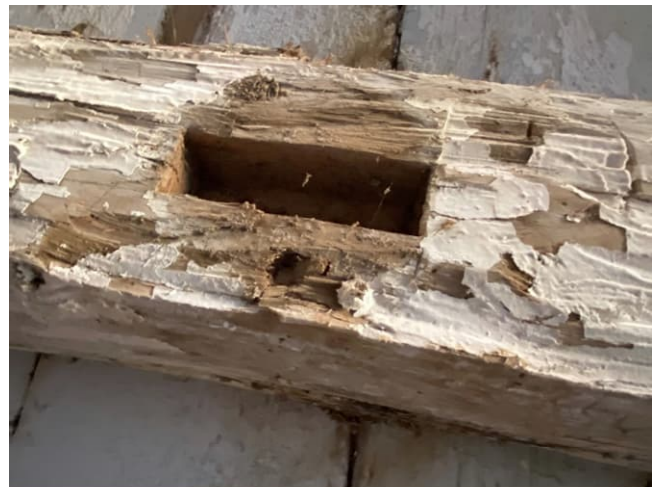
Plate 83: Redundant mortise in hand hewn floor joist
