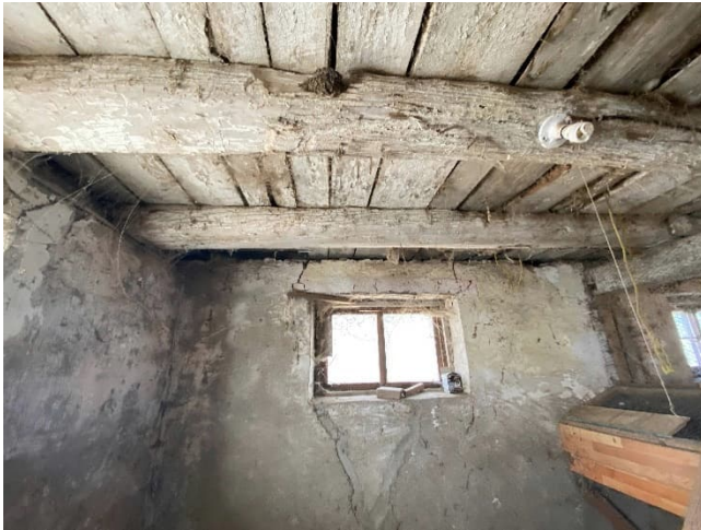
Plate 88: Parged wall with window
