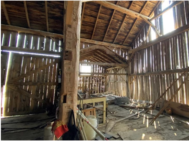
Plate 102: Post with redundant mortise
