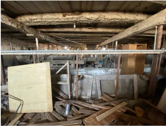
Plate 76: View of livestock stalls. Looking north from the south end of the centre block
