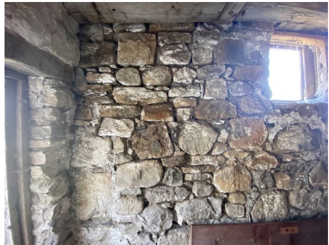
Plate 79: Stone foundational wall constructed with a mix of roughly dressed stone and rubble fieldstone
